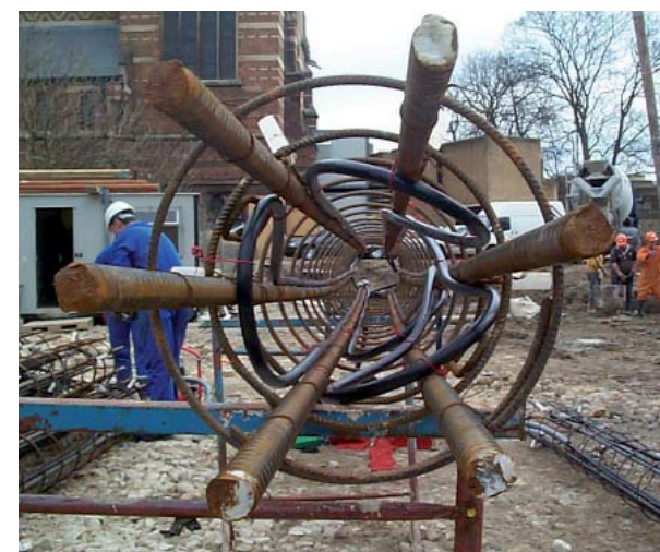
Geothermal pile structure at Keble College
