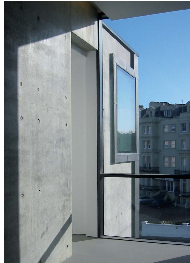
Exposed concrete helps to control and reduce rapid temperature fluctuations in the new Towner gallery
